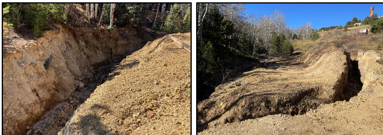
Figure 11. Site #136 - Channelized and incised section of Willis Gulch ~ 450 feet downstream of waste pile (left) and gully erosion of mine waste adjacent to Willis Gulch ~ 400 feet downstream of waste pile (right).
