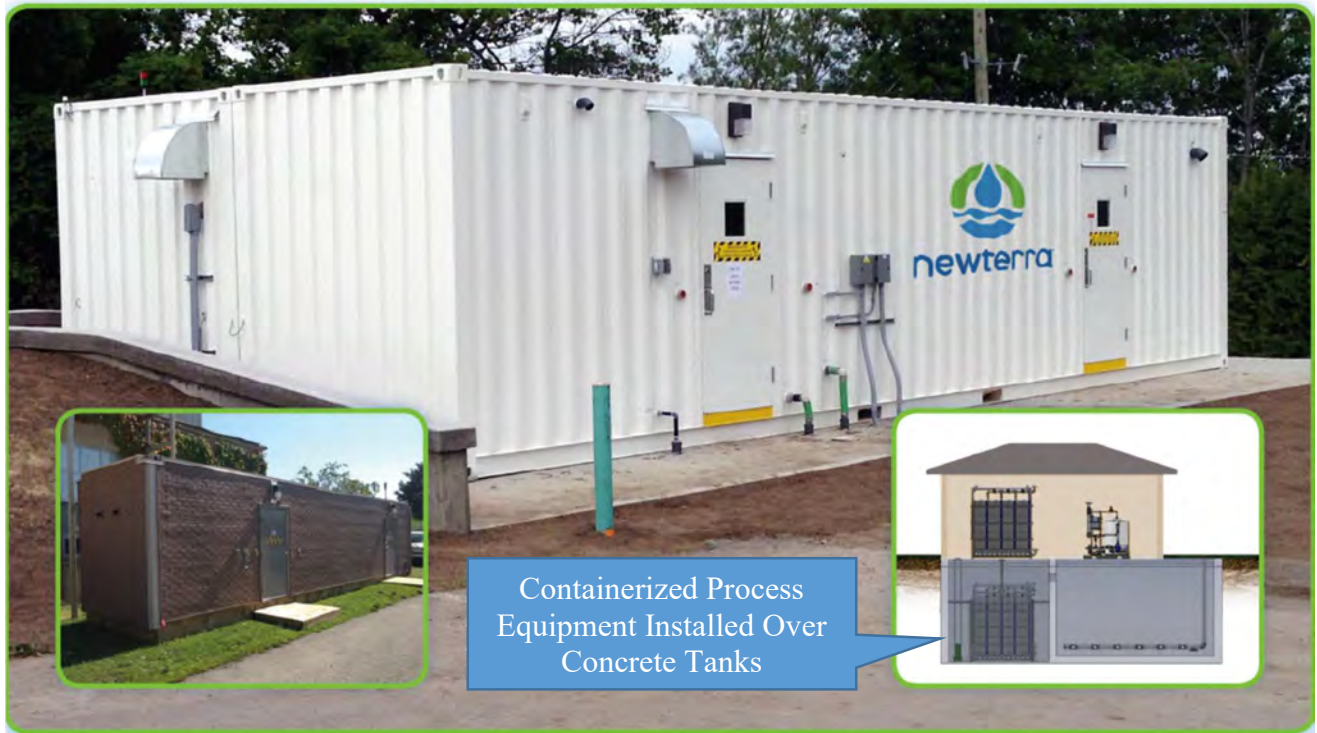
Figure 16: Newterra Containerized MBR System
