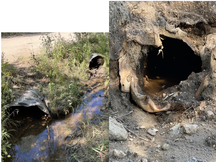
Figure 2 & Figure 3. Current culverts at the upstream section of Missouri Creek off Missouri Creek Road
