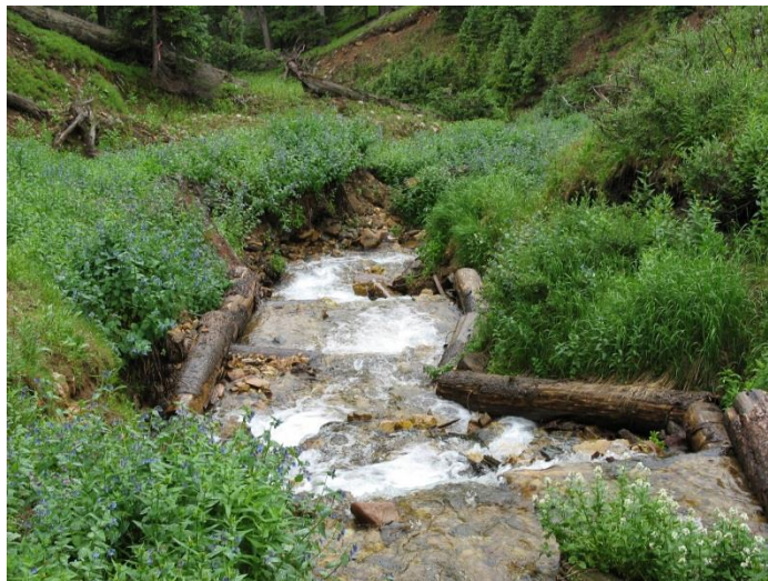
Figure 4-9: Berthoud Pass channel bank stabilization showing downstream erosion July 27, 2007
