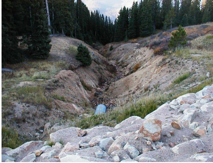
Figure 4-7: Berthoud Pass Ditch discharge channel showing massive soil loss September 25, 2001
