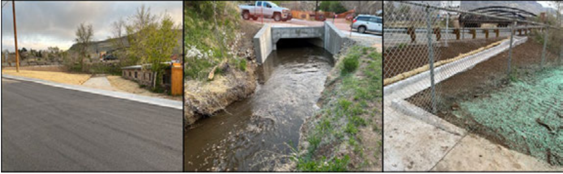
Left: Arapahoe culvert replacement and extension, middle: Arapahoe culvert inlet, right: Highway 52 exit ramp storm water diversion channel
