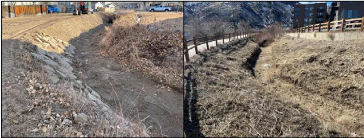
Left: Vegetation removal, ditch shaping, and rip rap placement to reduce erosion near W. 75 th Way, right: Vegetation removal Basecamp in Golden
