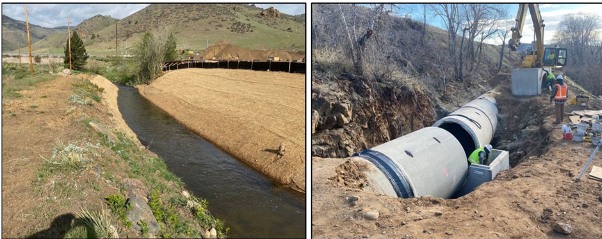
CDWA and the Basecamp Development infrastructure work on the Church Ditch (left) and a pipe installed for the Peaks to Plains Project (right)
