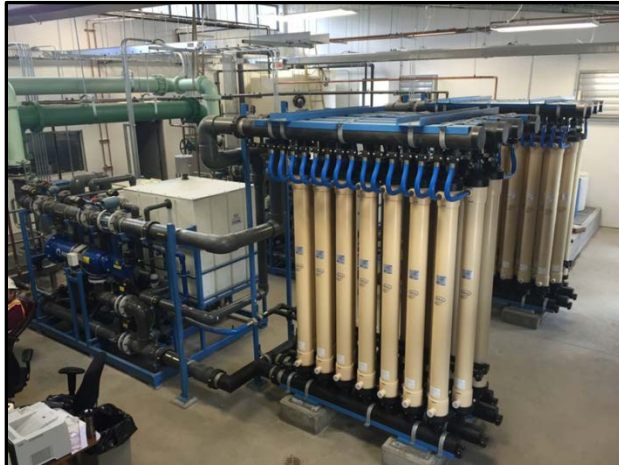
New Microfiltration System at Dory Hill Plant
