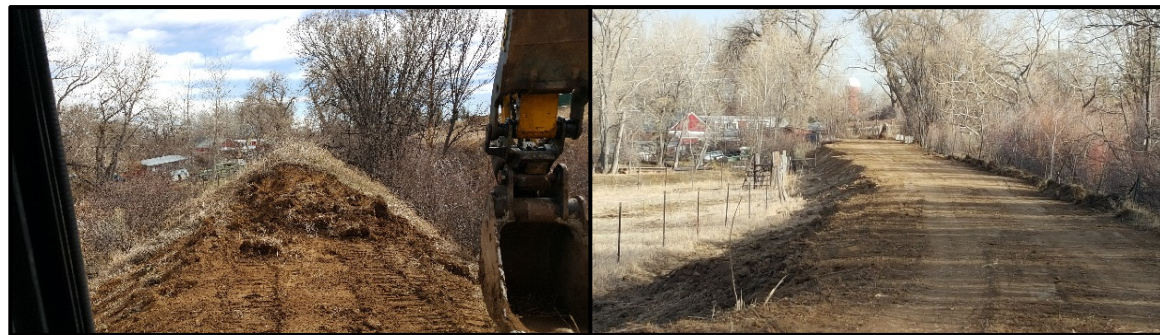
Building New Access Road Along the FHL, Before (Left) and After (Right) Construction.
