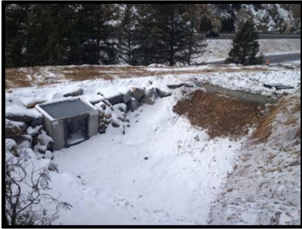
Rough Grade of the Hoosac Gulch Sediment Removal Basin and Inlet Box (Photo Credit: CCWF)
