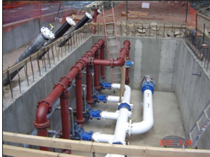
Figure 21. Hidden Valley Water Treatment Plant Infiltration Gallery
