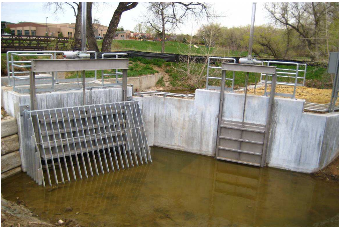
Figure 27. New Church Ditch separator at Little Dry Creek. Ditch is diverted under Little Dry Creek through the structure on the left. The sandout gate on the right returns water to Little Dry Creek in the background.
